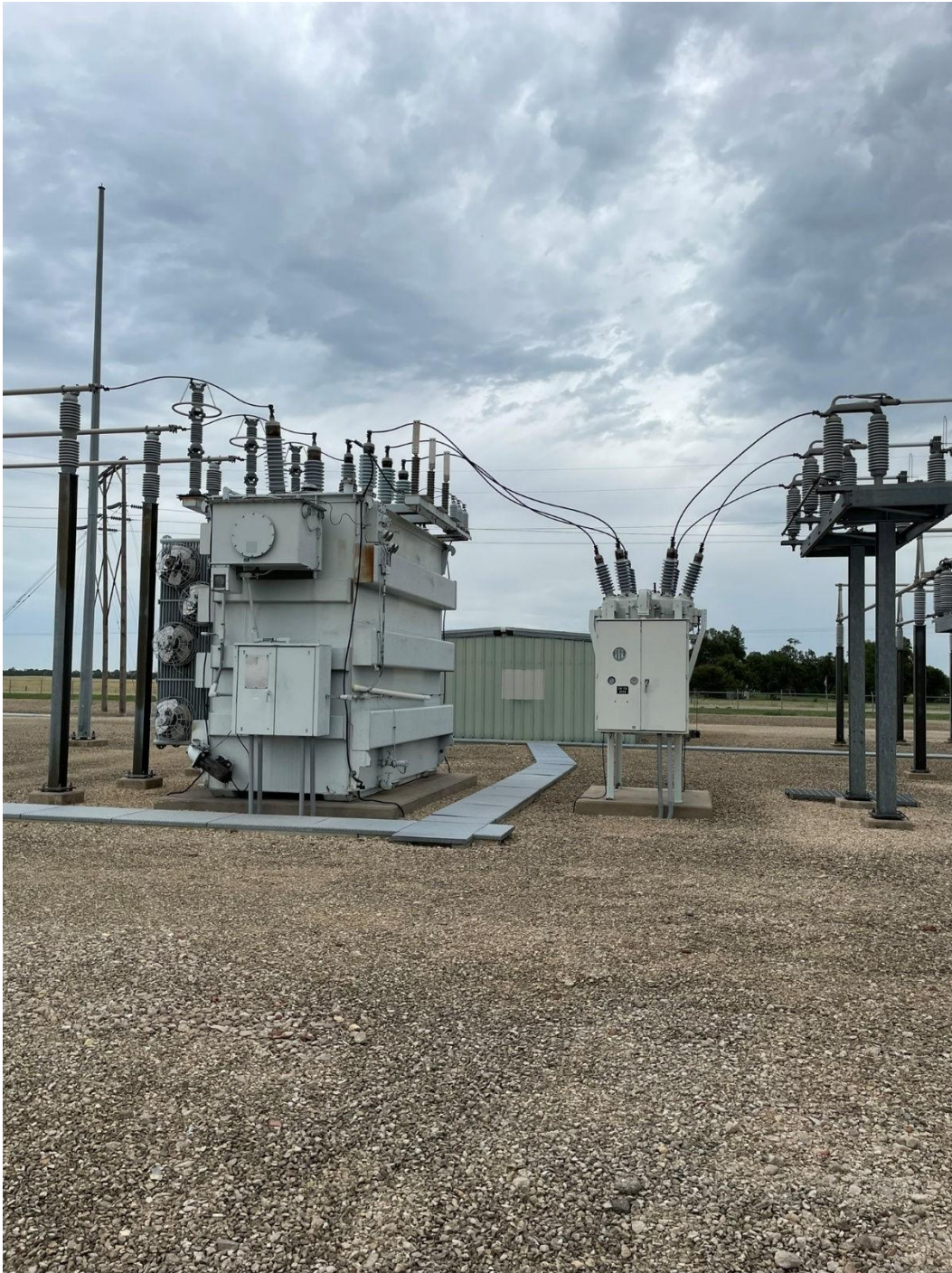
Figure 1: Seward 115kV/69kV Transformer and Cable Trench
